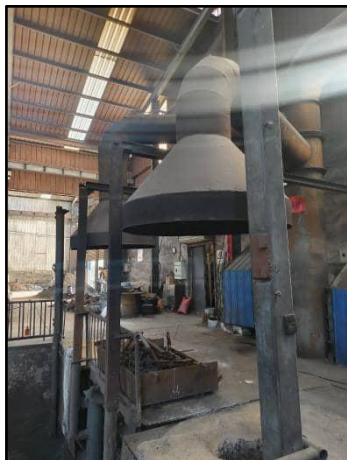
现有中频炉废气收集设施
